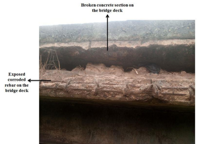
Figure 14: Visible signs of severe deteriorations on the section X of the Orogodo Bridge Deck
