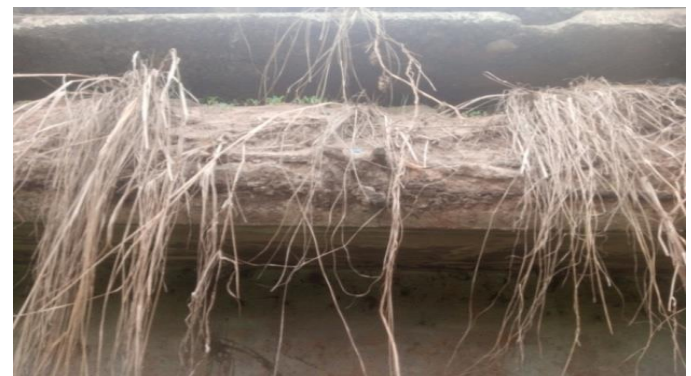
Figure 15: severe broken concrete section with dried vegetation an exposed corroded steel rebar
